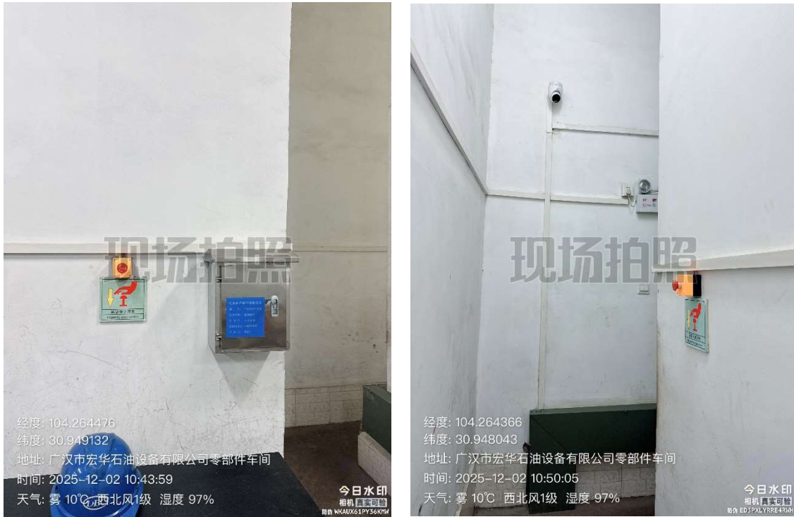
(a) 探伤内墙上紧急停机按钮
